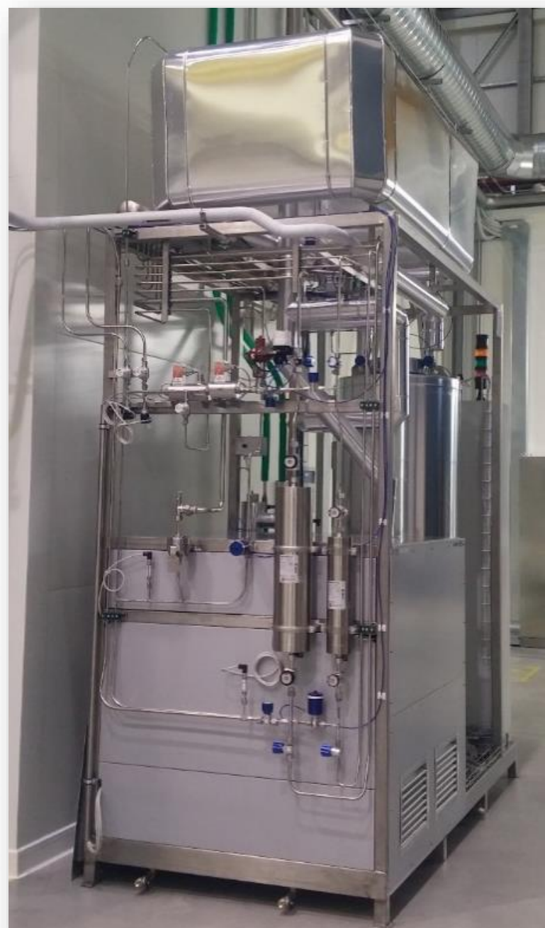
CO2 Purification system at ppb level for ExoMars Space Mission
