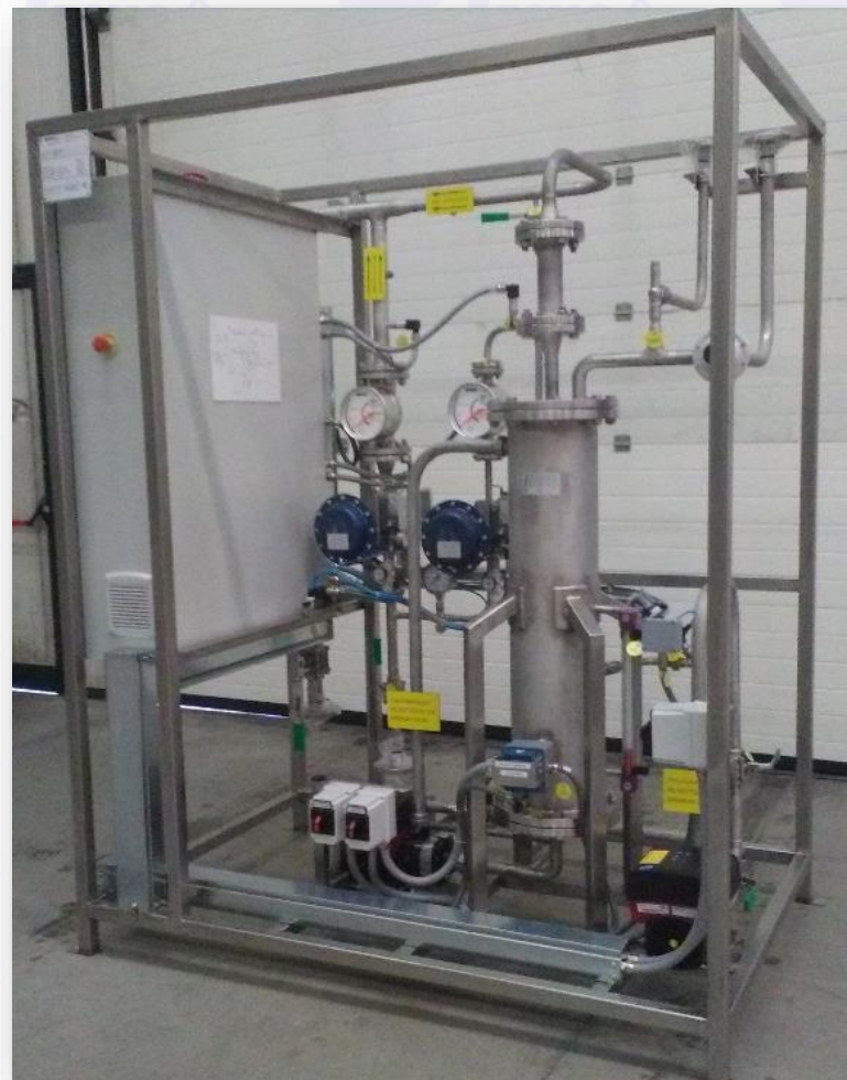
Nitrogen wetting system
